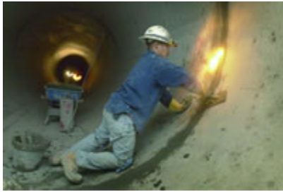
Aber Samaniego caulks the joints of a 108-inch-diameter pipe that will carry irrigation water to the western end of the Gila River Indian Community. Mark Henle/The Arizona Republic water.
